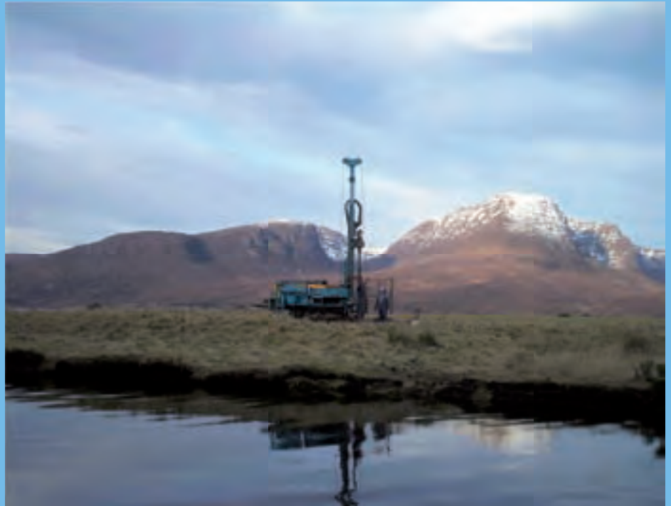
Boart Longyear DB520 rotary rig using ODEX system to drill through coarse, granular deposits near Kishorn, Scotland
